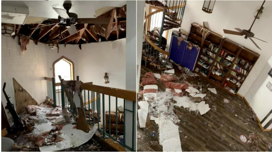
(Figure 1: Busted water pipes and damage during the storm)
